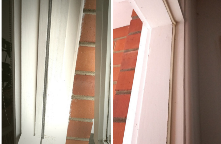
Figure 5: Grey seal (left) and white seal (right) used to reduce draught from windows
