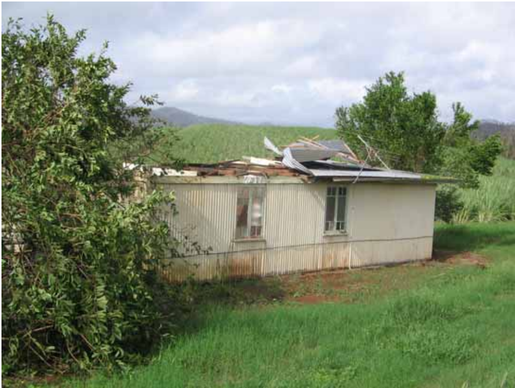
Photograph 1: Housing damaged in Innisfail Queensland 2006
