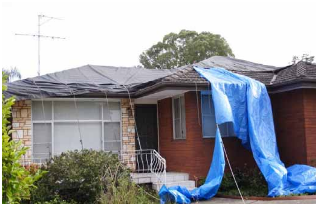
Photograph 5: House damaged in Blacktown NSW 2007
